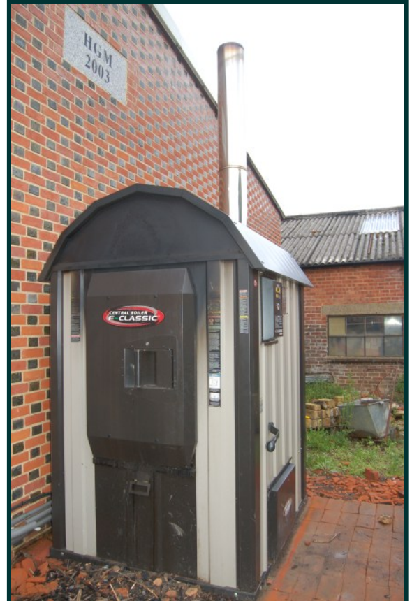
Wood boiler unit at Bellingdon Brickworks
