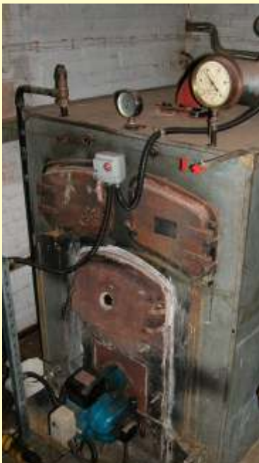
Oil boiler due for replacement
