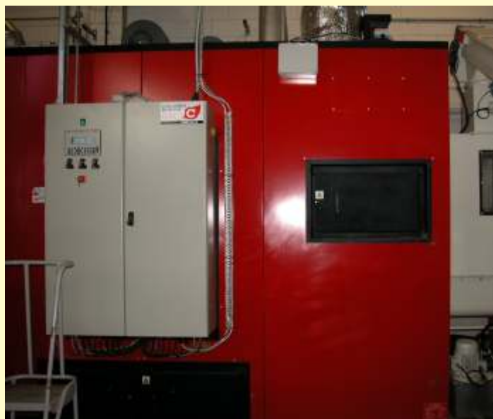
New wood fired boiler
